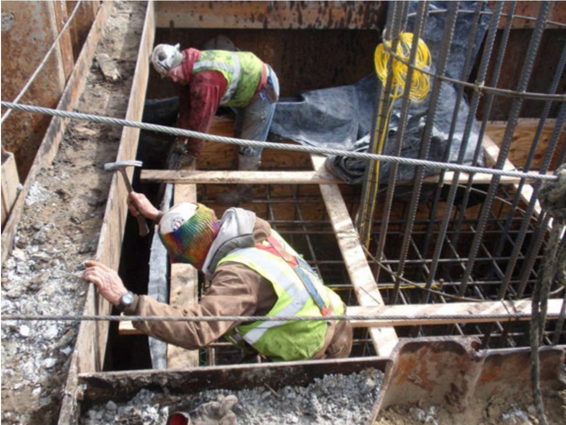
Figure 2.6 Insulation being installed on the outside of the formwork of a mass concrete placement
