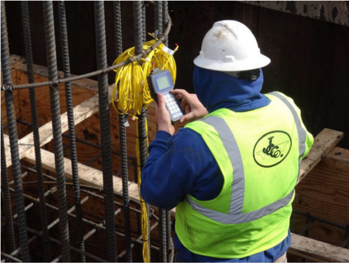
Figure A.6 Verification of proper sensor function after installation
