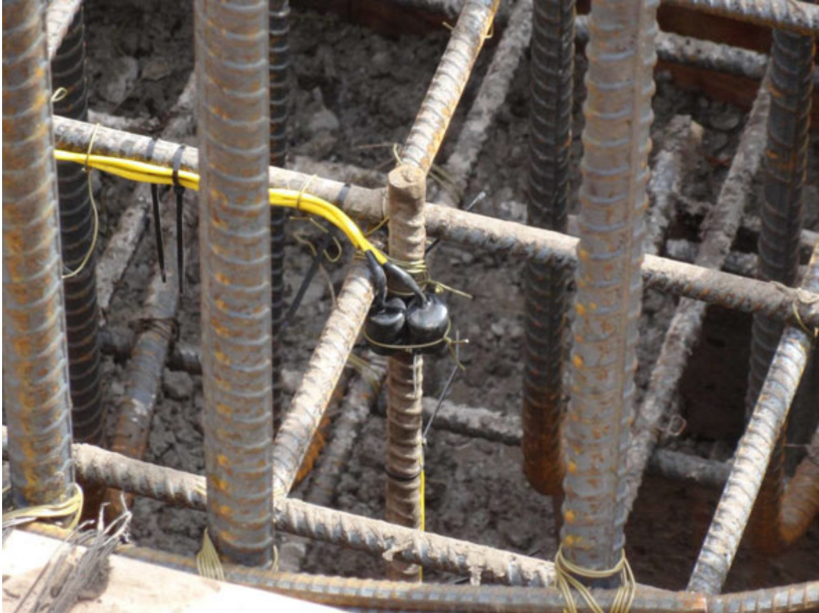
Figure 2.12 Installed thermal monitoring sensor
